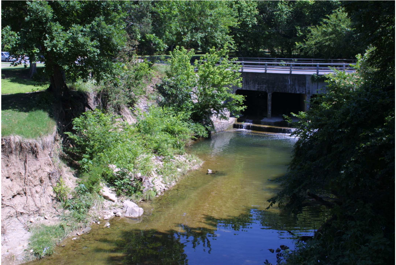
View looking south to Colorado bridge – May 2003 showing: solid paved foundation, rock filled galvanized wire basketry stepped down the bank immediately beside the bridge, and a large tree threatened by ongoing creek bank erosion
