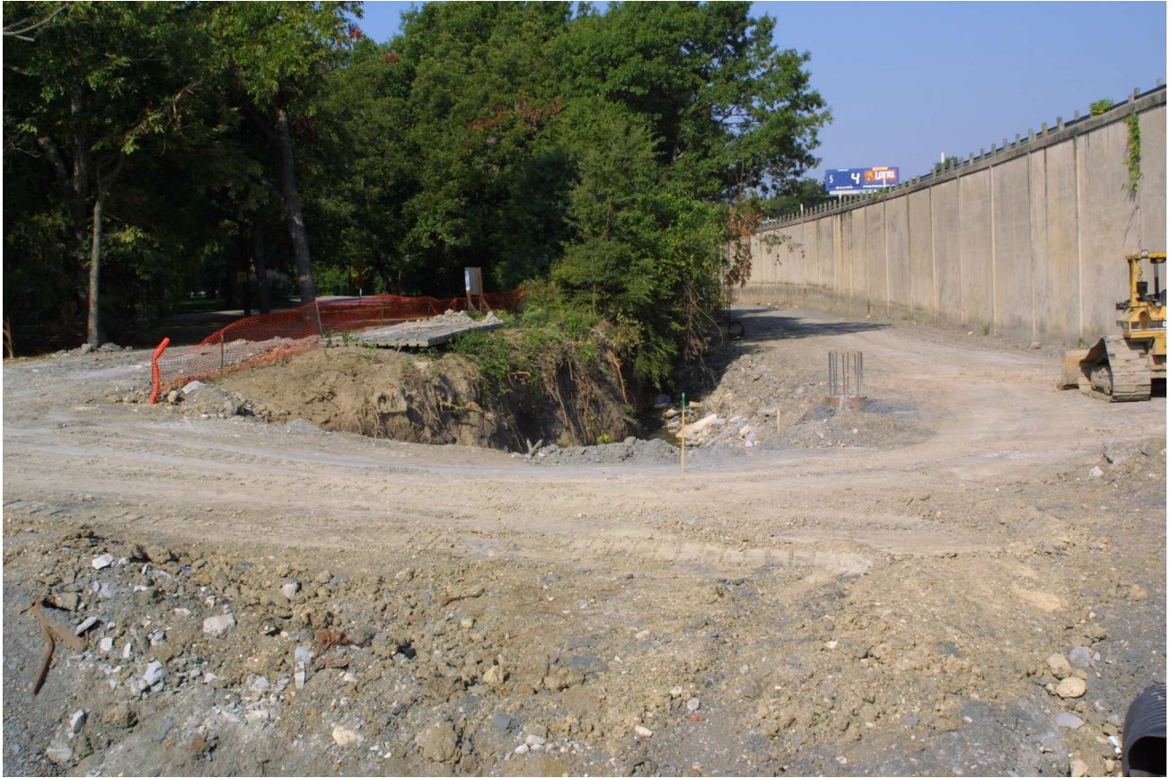
New Interstate 30 widening just above Sylvan –to extend two new lanes of highway construction cantilevering over the creek — August 2003
