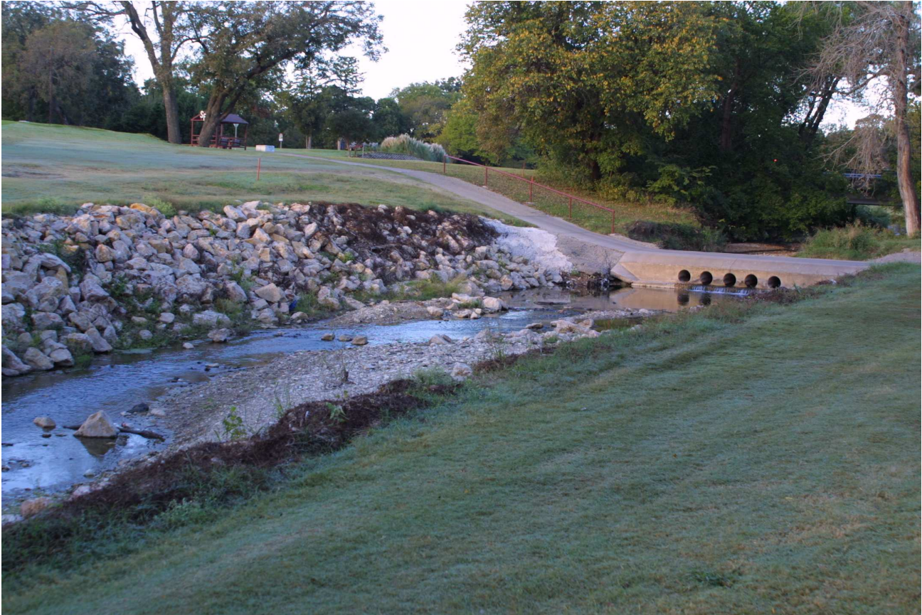
Just below the North Oak Cliff Boulevard bridge, large loose boulders of Austin limestone have been dumped along the banks. Raw concrete has been dumped at the end of the cart bridge to try to stop scouring by floodwaters. --- October 2003
