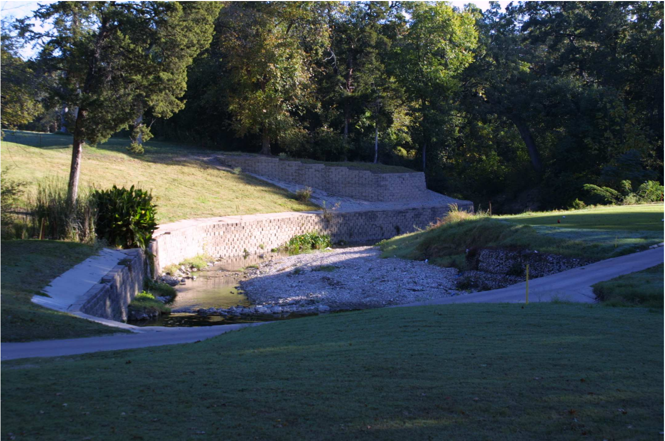
Concrete block walls on the left bank below the North Oak Cliff Boulevard bridge --- October 2003
