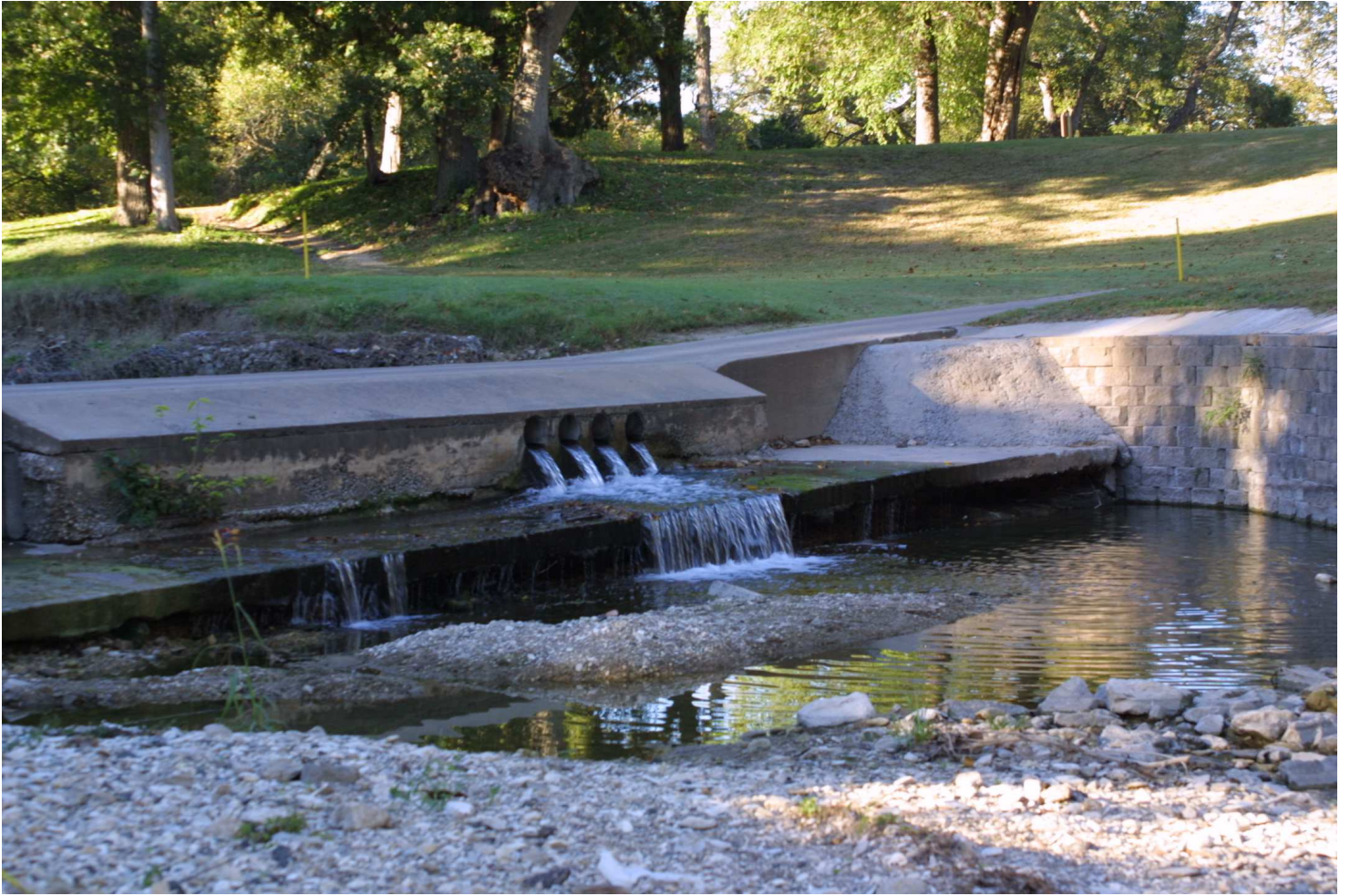
Cart bridge being undercut by scouring -- downstream from N. Oak Cliff Blvd. bridge --- October 2003
