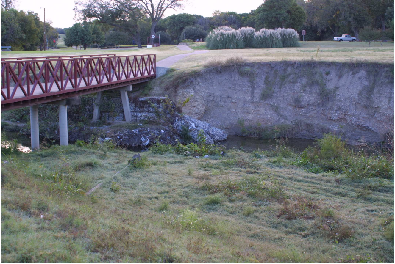
View looking south between Hampton and the North Oak Cliff Boulevard bridge, showing cart bridge that has been shored up with loose rocks behind galvanized wire basketry. Extreme new erosion can be seen to its right --- October 2003
