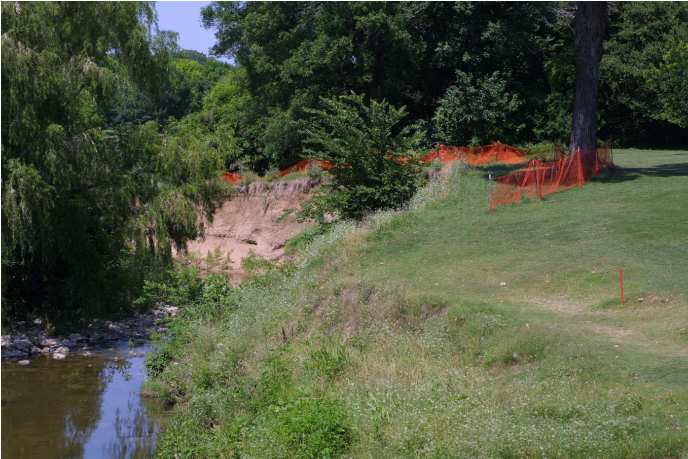
Portion of the creek bank very near failing, just below the Colorado bridge — May 2003
